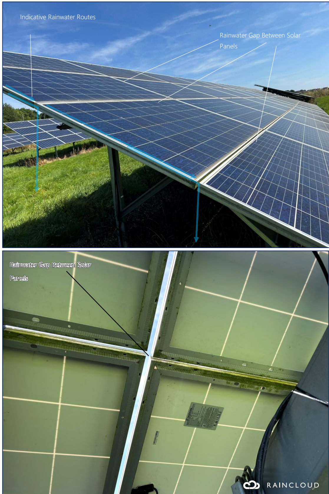
Plate 12-25 Rainwater gaps on PV array table
