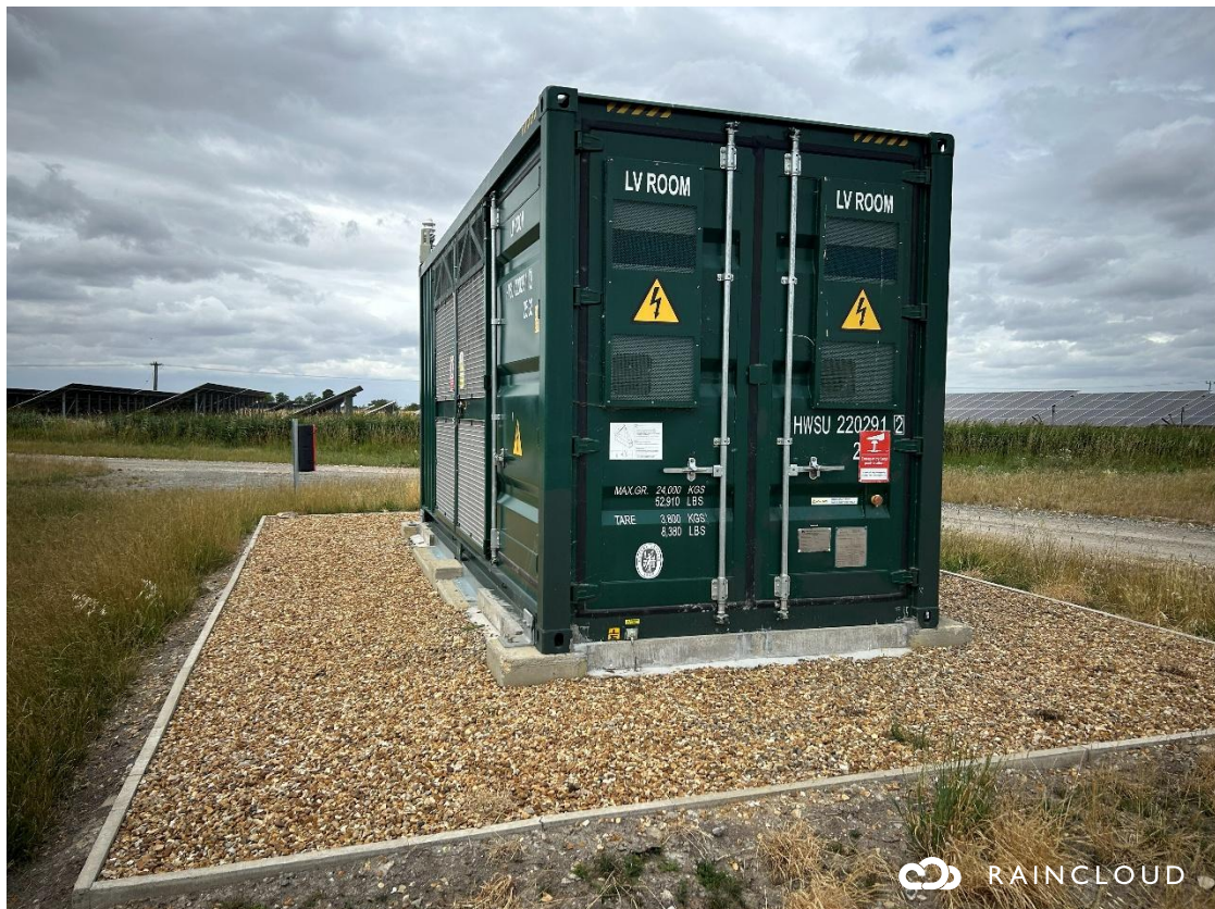
Plate 12-33 Conversion unit gravel surround
